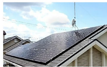
太陽光発電設備 Solar power generating facilities
